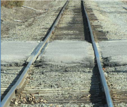
The Project will rehabilitate existing track, including rail, ties, ballast, spikes, anchors and tie plates
