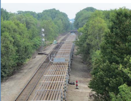
Continuously welded rail will replace existing jointed rail to reduce maintenance costs and provide a superior ride quality for passengers.
