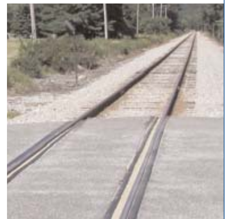
36 Grade crossings will be upgraded to the standard pictured above, providing a smoother transition for trains and motorists alike.
