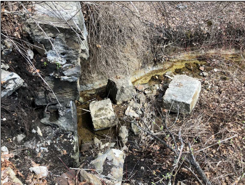
Photo #10: Three Stones from Failed Outlet Headwall/Wingwall in Channel
