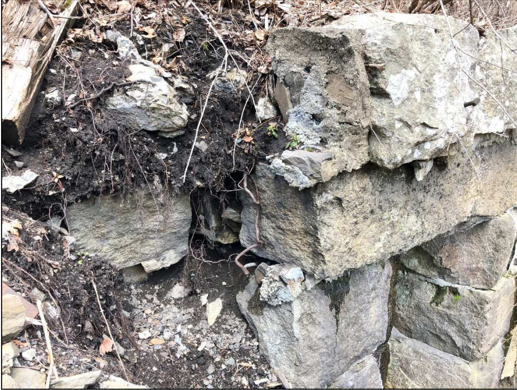
Photo #9: Failed South Wingwall and Headwall at Outlet
