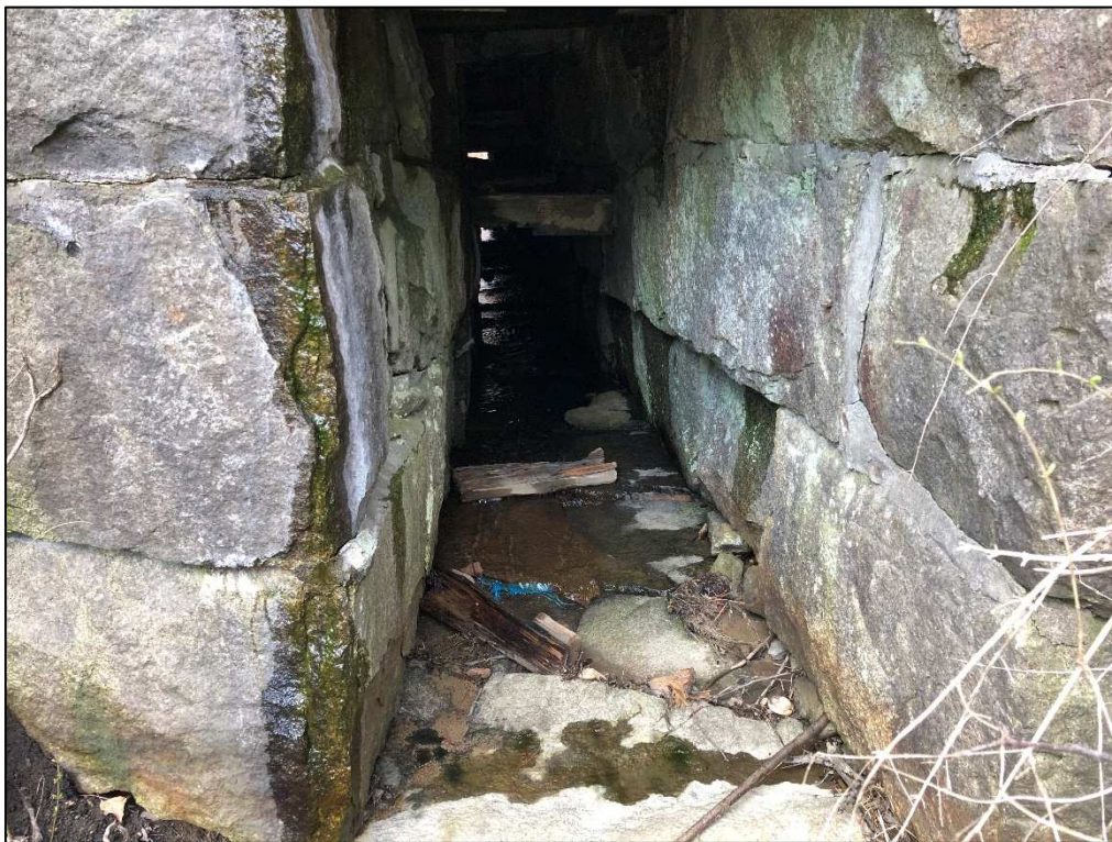
Photo #8: Undermining of Stone Culvert Floor Allows Flow Under Culvert at Outlet
