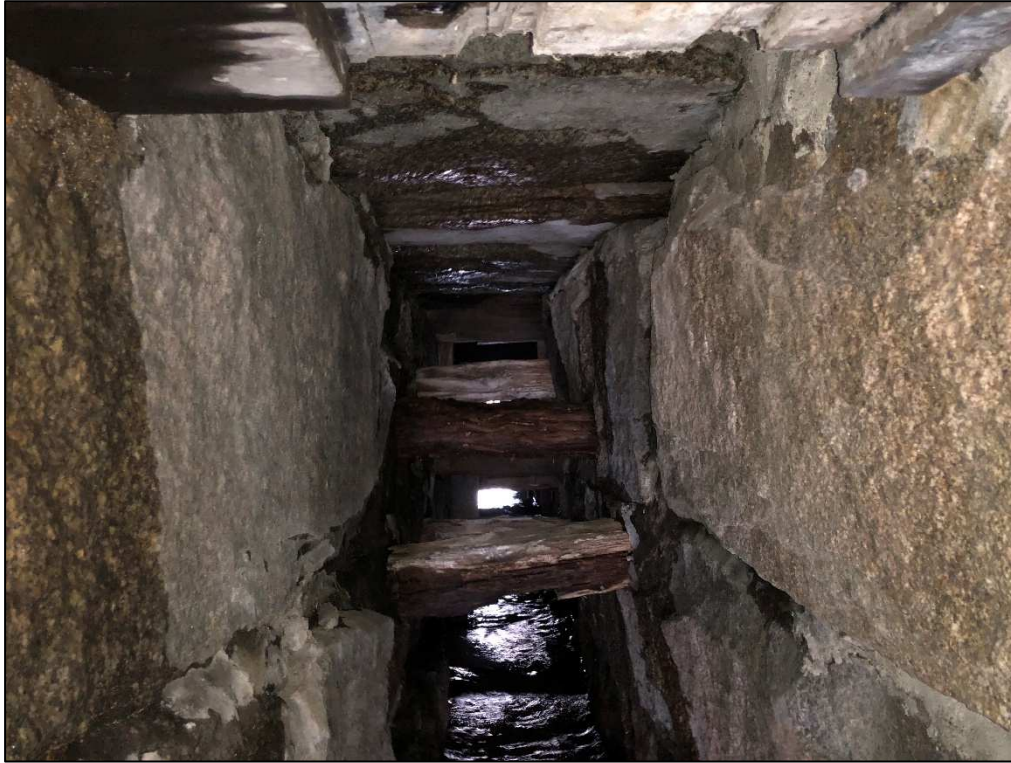
Photo #7: Horizontal Opening of 4' Reduces to Approximately 18" – Approximately 30' From Outlet
