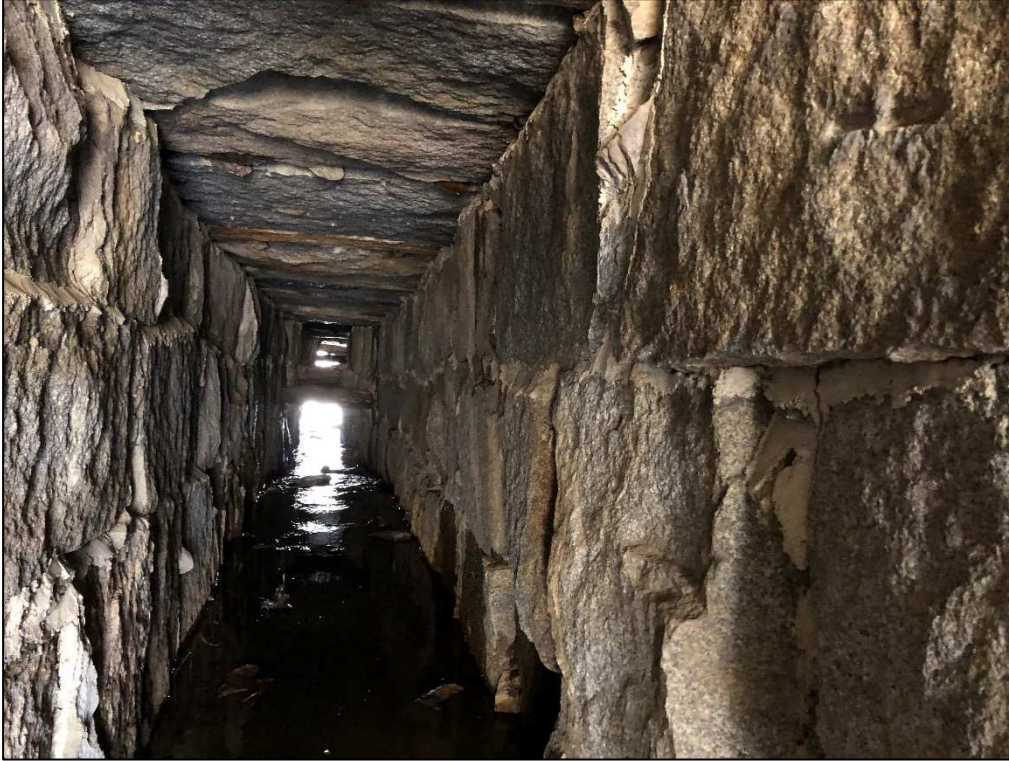
Photo #5: Stone Box Culvert in Good Condition for Approximately 40 Feet From Inlet
